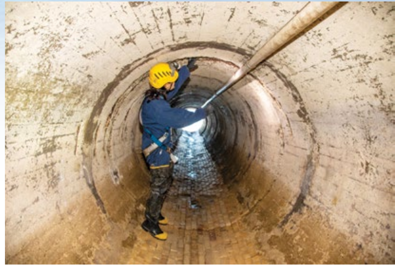
Major projects include replacing approximately 1 to 1.5 miles per year of old brick sewer trunk lines
