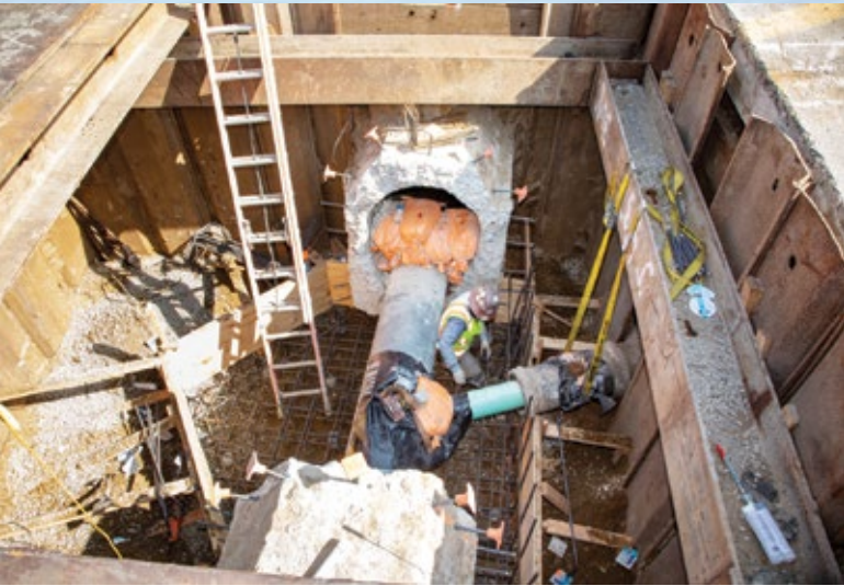
15 miles per year small diameter gravity sewer rehab/replacement work using trenchless construction
