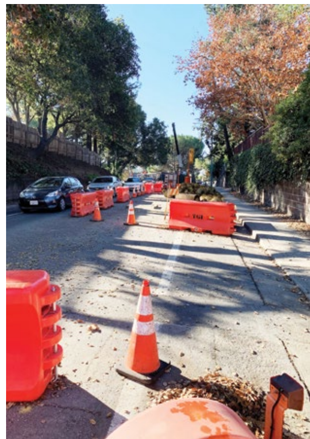
A mature area of the central city made limiting the size of the job site footprint critical
