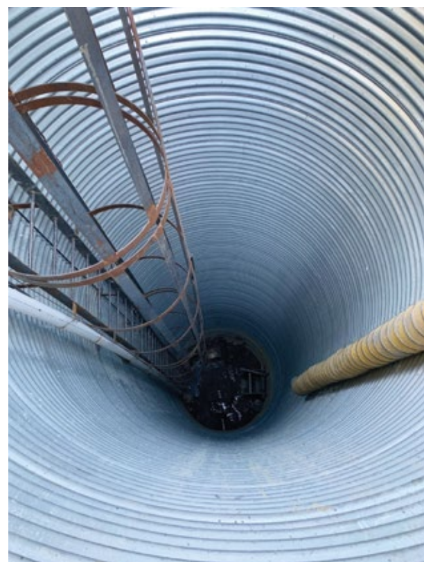
Shaft diameters of 12 feet or less and depths of up to 40 feet made this installation possible
