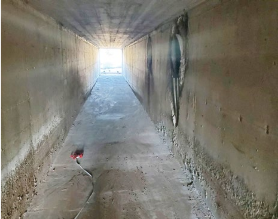
Box culvert had failing concrete and exposed rebar
