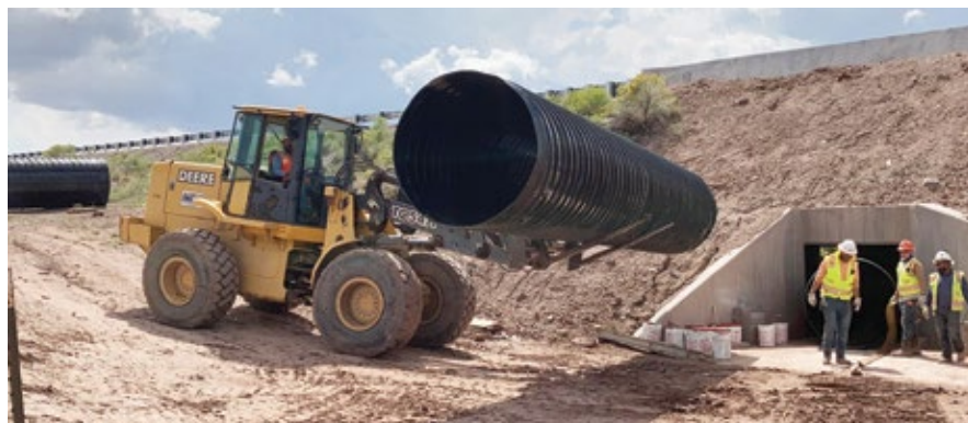
Pipe is so light the contractor was able to use a medium-sized front-end loader to move each segment
