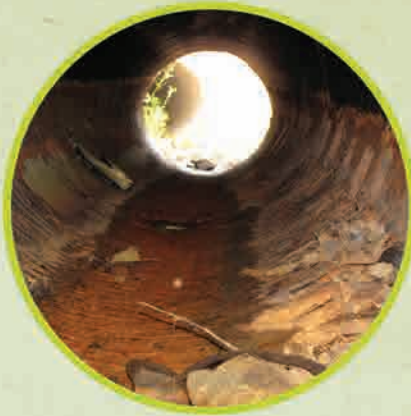
BEFORE CORROSION & DEBRIS CREATE INFRASTRUCTURE INSTABILITY
