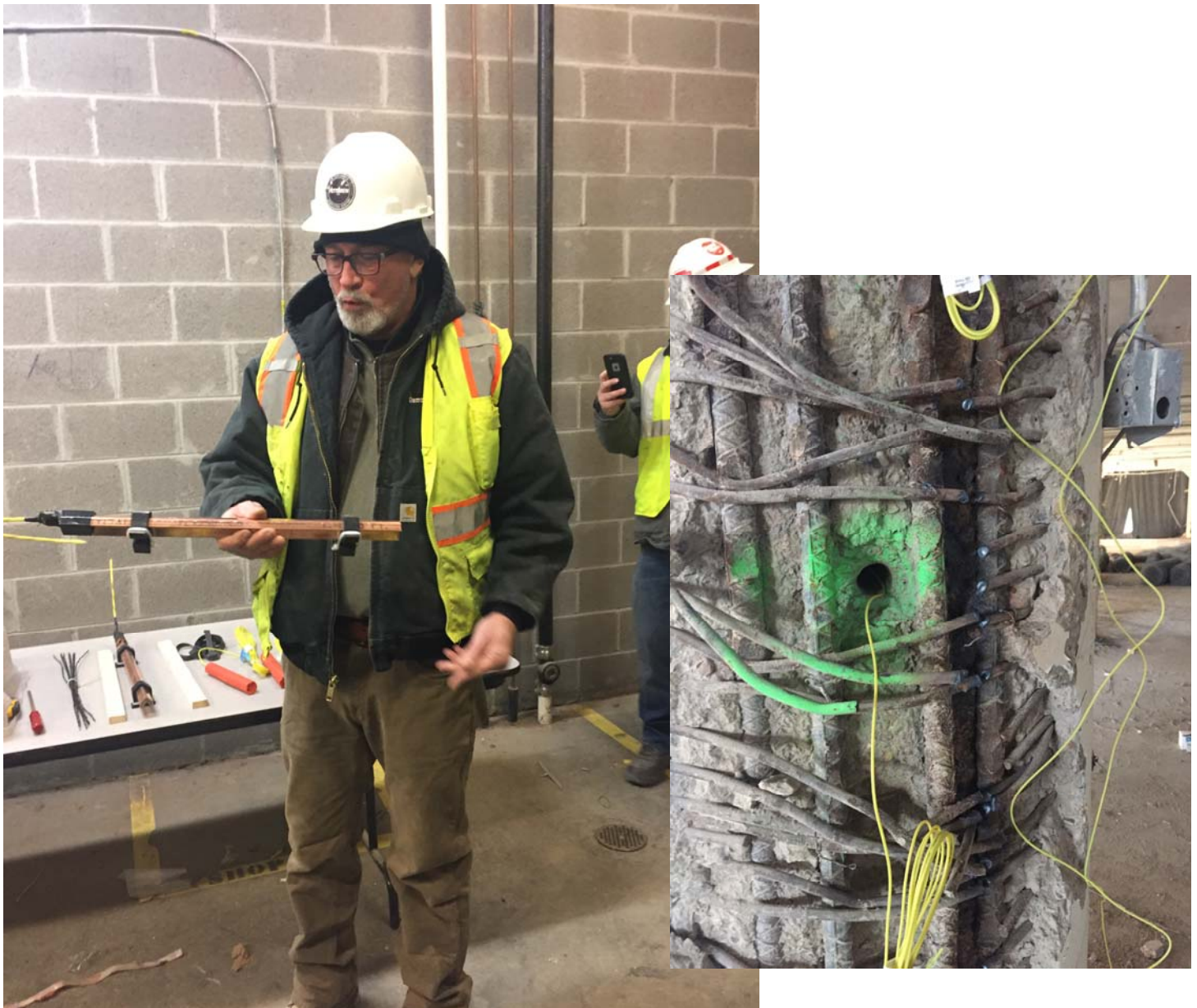
Explaining to students how the charges are laid out for demolition of existing building National Museum of African American Music, Skanska, Aug 3, 2018
