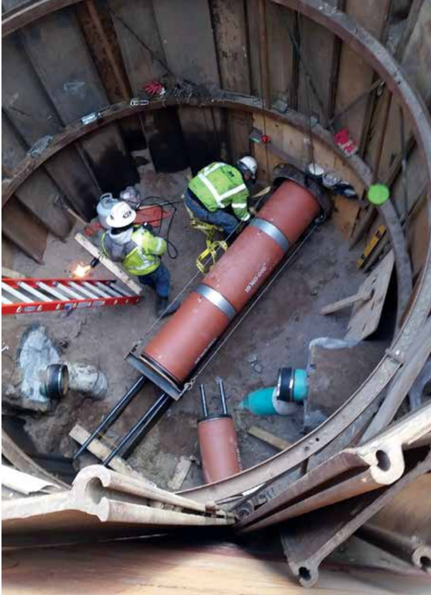
Minger Construction used a variety of shafts at depths of up to 20 feet
