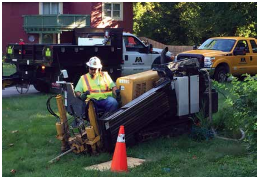
HDD allows pipes to be installed with few public impacts and inconveniences to homeowners
