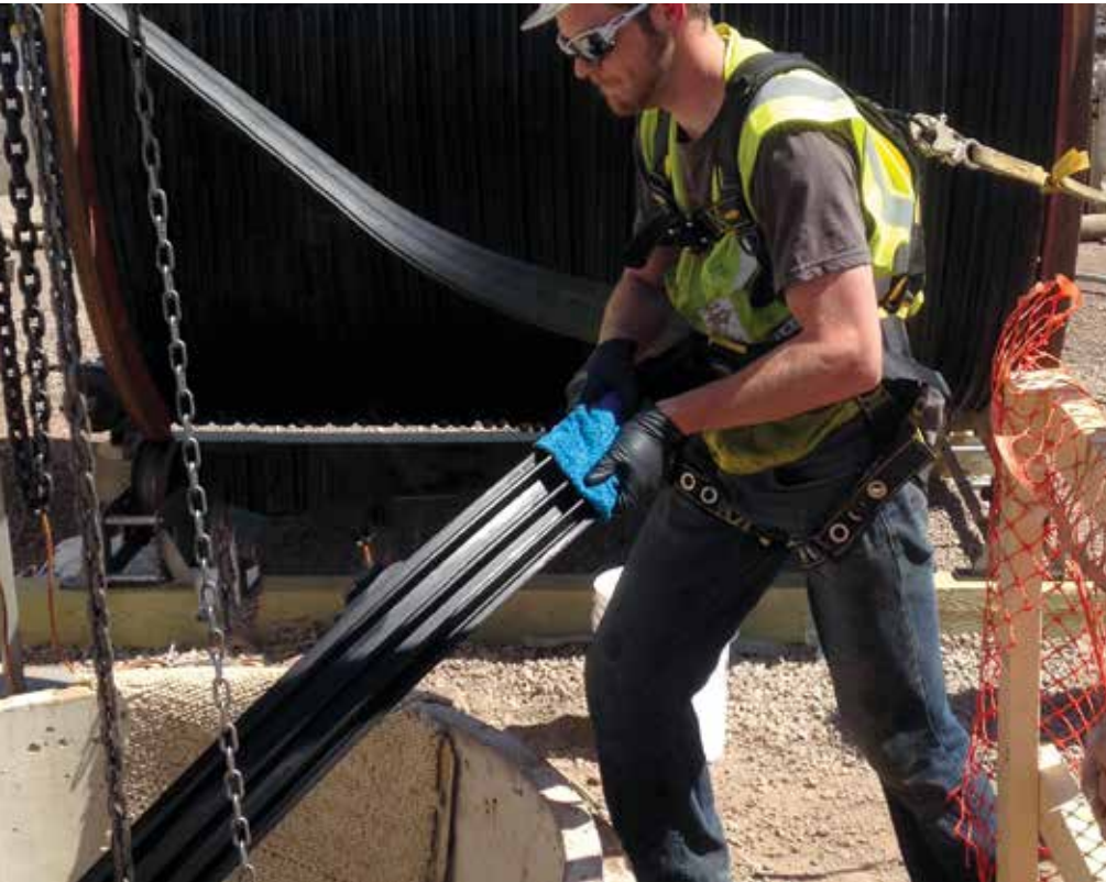
A single strip of steel reinforced HDPE profile was progressively fed into the winding equipment inside the existing pipe
