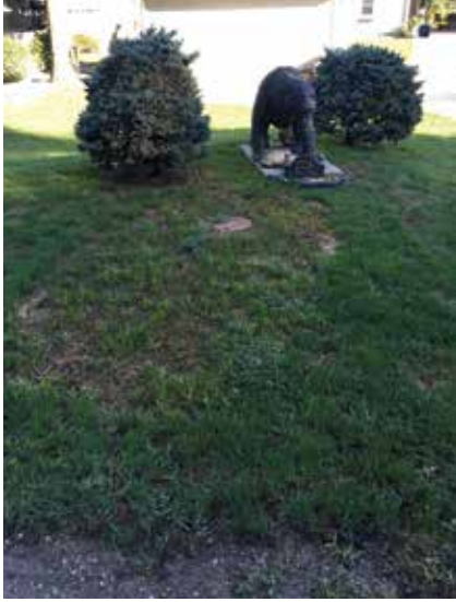
Installations are completed with minimal invasiveness and restoration done immediately. The general public has embraced the STEP program
