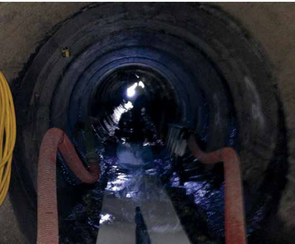
Thirty-seven feet underground, 394LF of new steel reinforced polyethylene pipe was manufactured in place.
