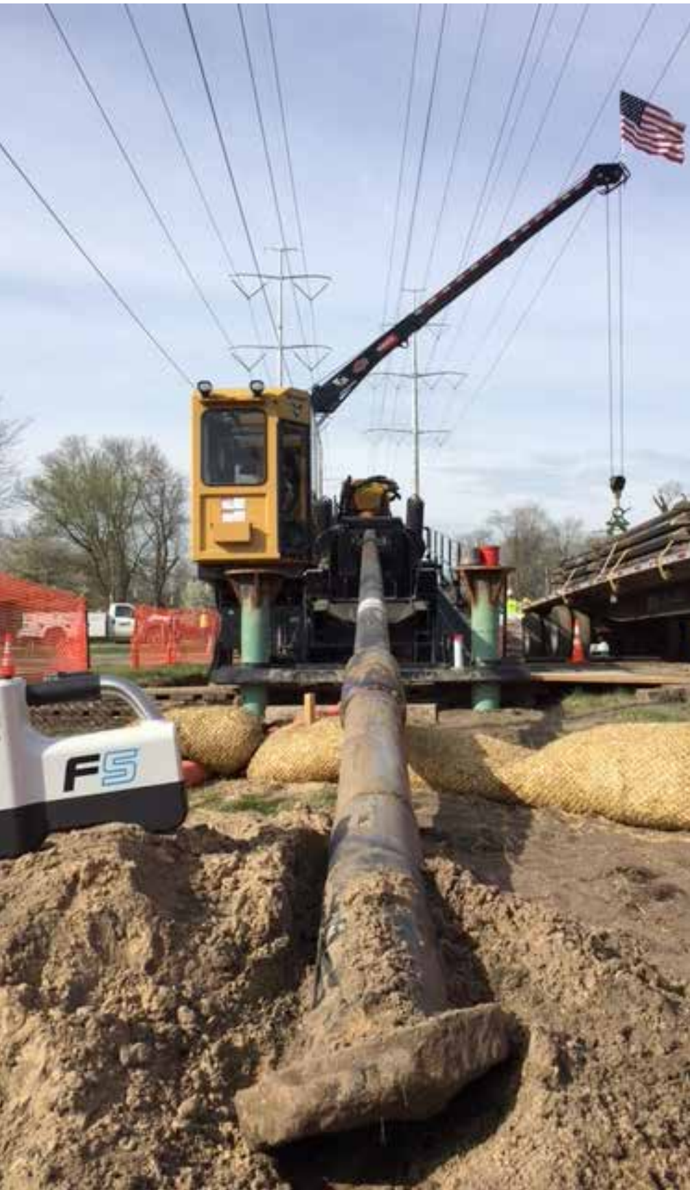
Using the Falcon F5 convinced the Bore Superintendent that the pilot bore could be completed with a walkover system
