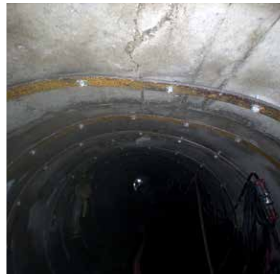
Structural steel banding was placed in the crown of the RCP in order to allow for safe work activity inside. The crown and invert had cracked due to excessive loads.
