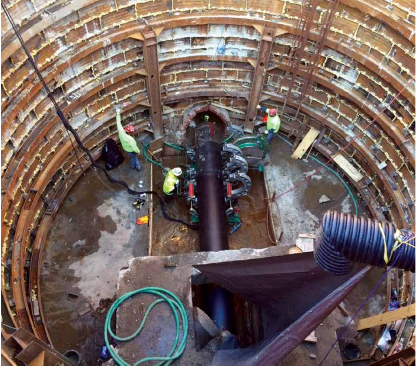
Installing HDPE pipe proved to be a well thought out and wise solution
