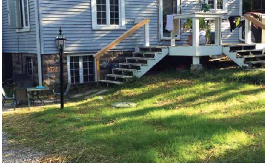
Post installation. Grinder pump lid is low profile, approx. 2 inches above ground
