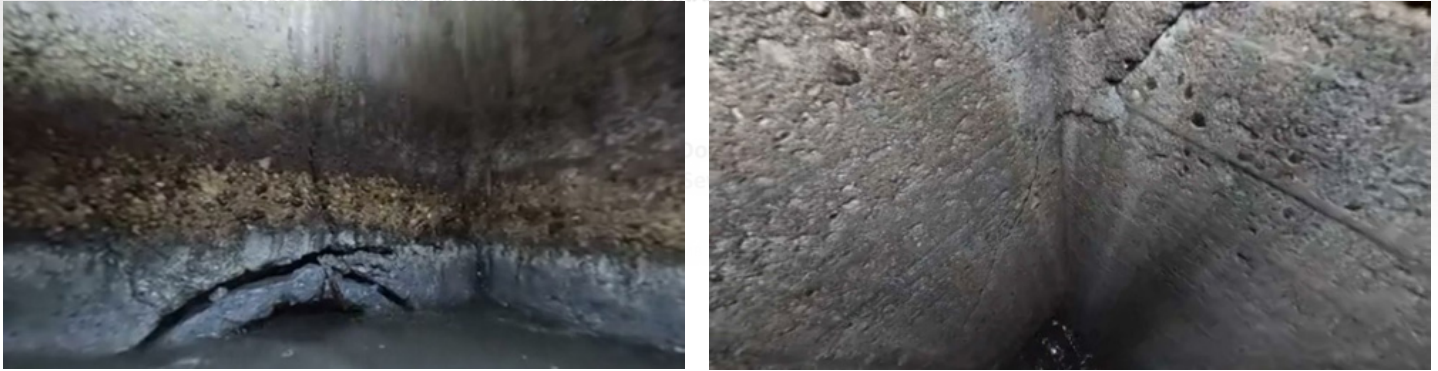
Figure 12. HCI Fractured Pipe (left) and Diagonal Fractures in Wall (right) Due to MH Settlement
