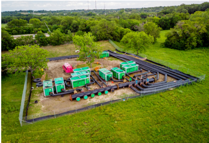
Figure 1 - 100 MGD Wet Weather Bypass
