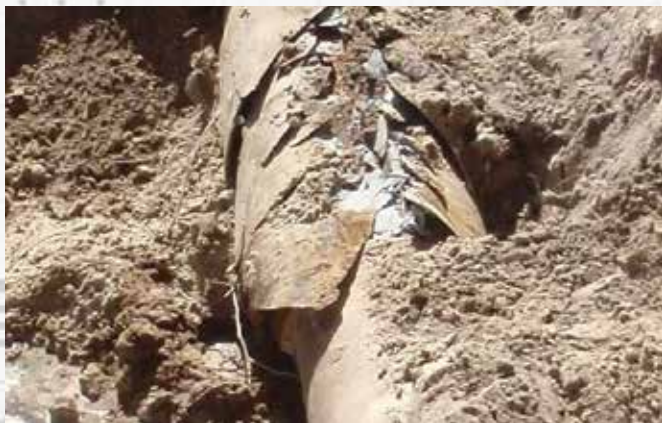
Figure 1 - Fractured AC pipe resulting from pipe bursting as it will remain in the ground.
