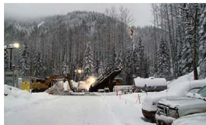
HDD intersect crossings on the banks of Wapiti River in Alberta, Canada.
