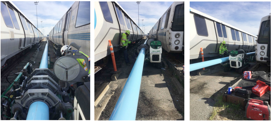
Pipe bursting was the most efficient method within a tight six-foot gap between tracks
