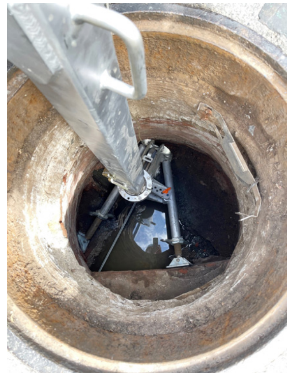
Cratus crews used a special reversible boom (pictured) for the pneumatic pipe bursting portion of the project. The boom creates additional space for detaching the busting tool from the winch cable in the manhole
