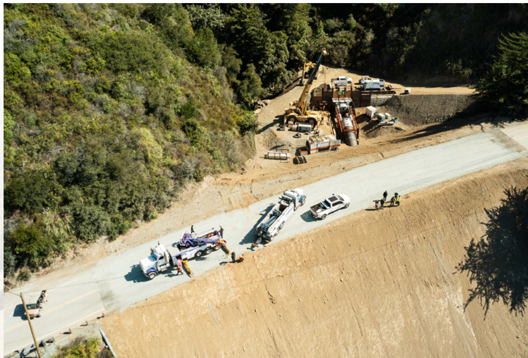
Installing 270 LF of 96-inch casing down a challenging -27% slope was a formidable challenge
