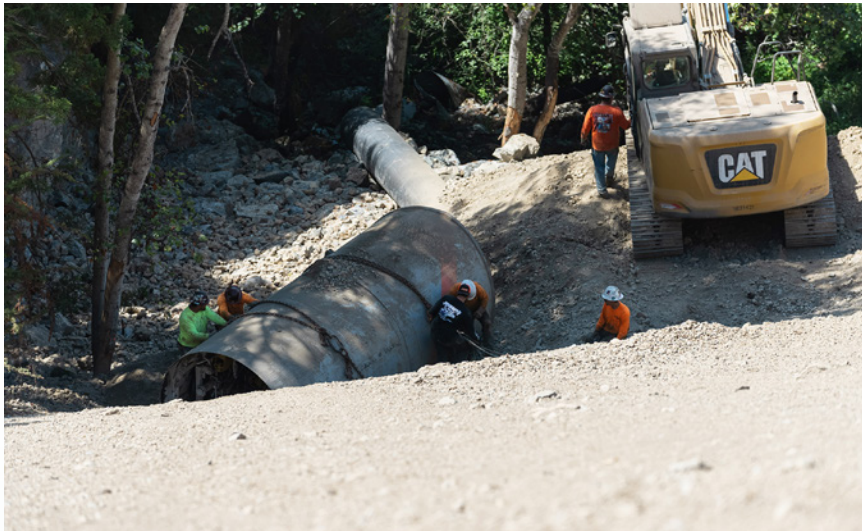
Failed culvert caused erosion and road collapse, shutting down a portion of Highway 1
