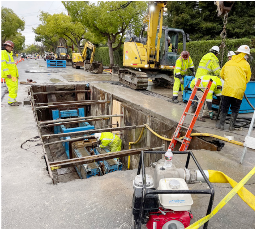
For a 700-foot section of 15-inch VCP to 18-inch HDPE, the Cratus crew utilized a Grundoburst 1250G static pipe bursting system from TT Technologies
