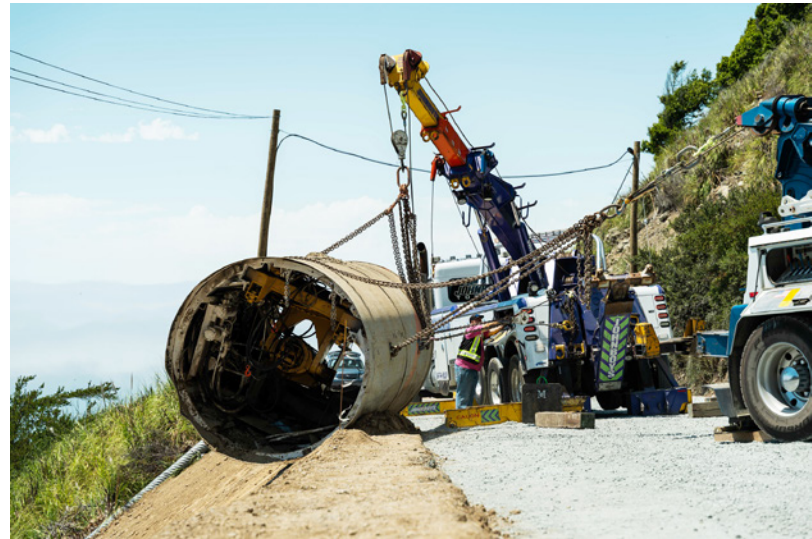
Two heavy duty wreckers were used to winch the boring unit back up the slope
