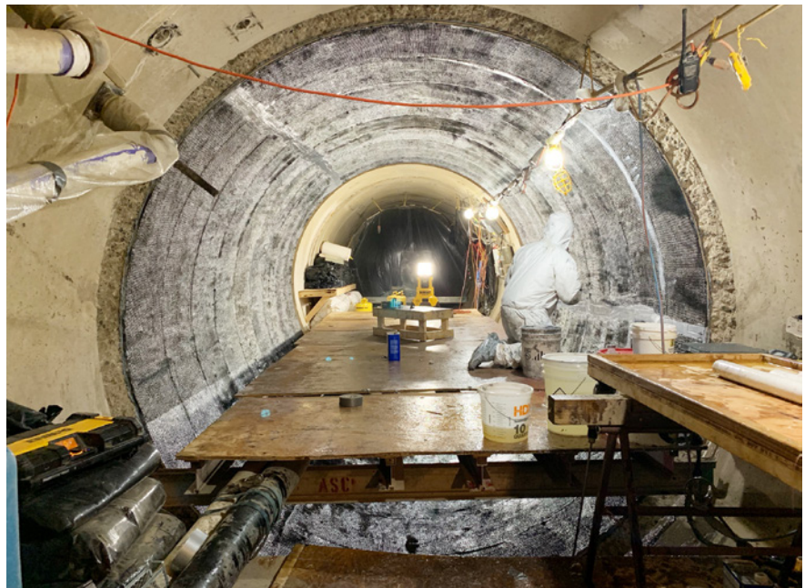
Figure 2. Fully-structural repair with the FRP composite system in a 100-foot deep tunnel in Minneapolis, MN
