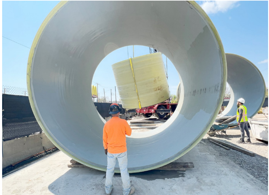
Figure 1. The record breaking, 16-foot FRP composite pipes being unloaded at the job site for installation
