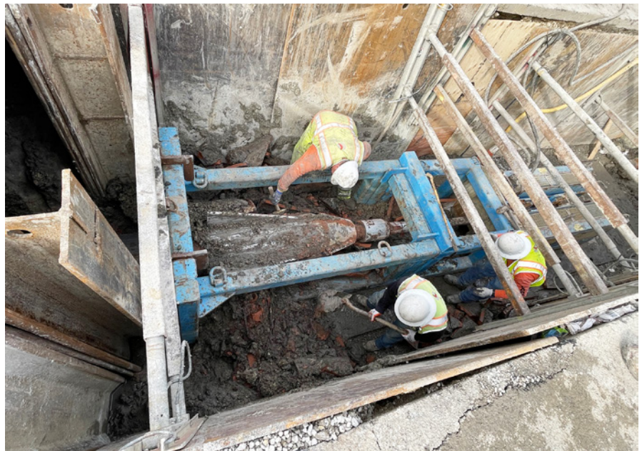
The Cratus crew proved proficient with both the pneumatic and static pipe bursting systems, successfully replacing over 10,000 feet of sewer main for the city of Palo Alto
