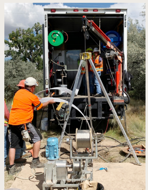
Typical compact set up above ground
