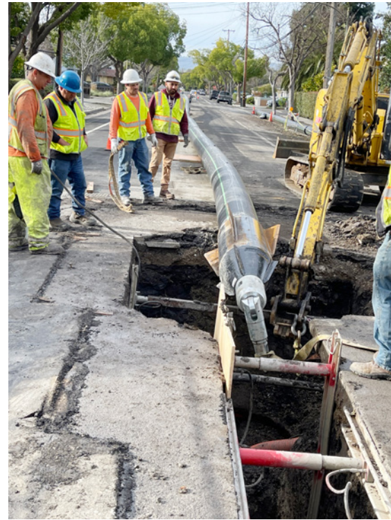
The 700-foot section of main was in an area near businesses and homes. The static system provided a quieter option than the large pneumatic hammer for that area
