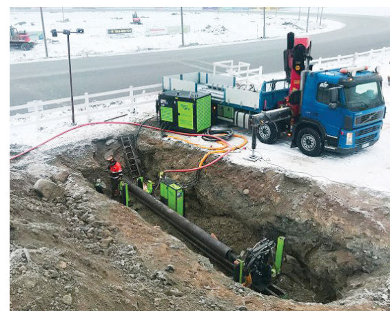
In Norway bores mainly run through strong to extremely strong 50,000+ psi unconfined compressive strength rock
