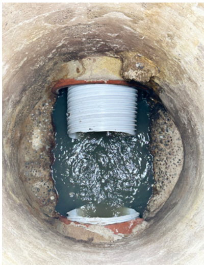
Result is a custom, tight fit liner with consistent wall thickness restoring hydraulic capacity
