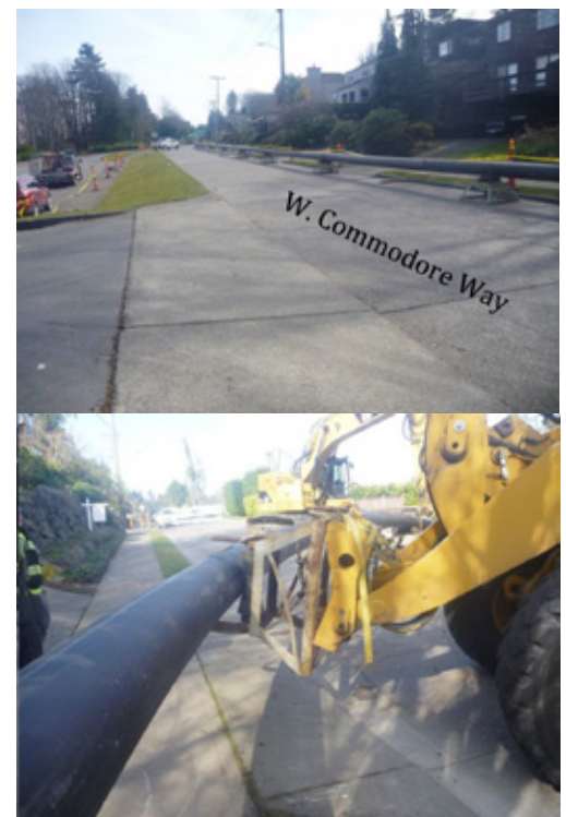
Figure 4: (Left) 16-inch HDPE pipe staged in roadway and (Right) Use of loader to manage pipe layout during pullback
