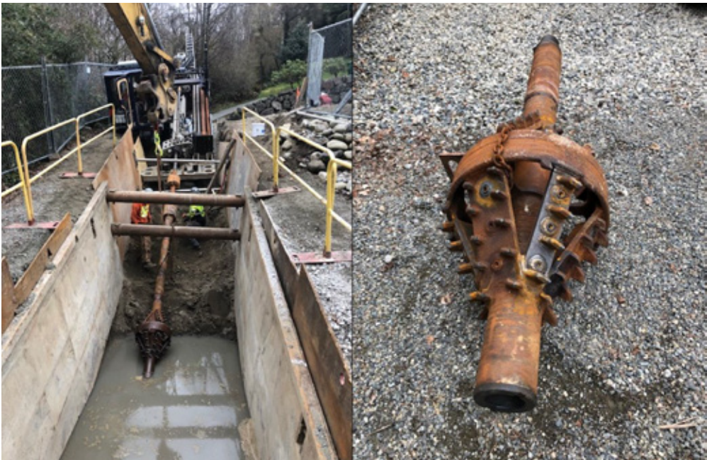
Figure 3: (Left) Ream Pass 1: 24-inch reamer installed on drill string and (Right) 24-inch Short Barrel Fly Cutter
