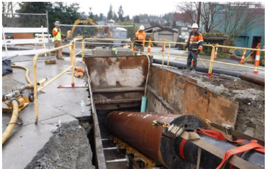
Figure 1: 20-foot section of 42-inch steel casing setup on guide rails and 20-inch pneumatic hammer
