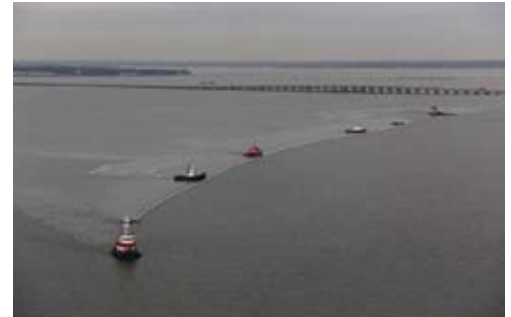
Figure No. 3 – Tug boats managing the product pipe as it is moved into position for pullback.
