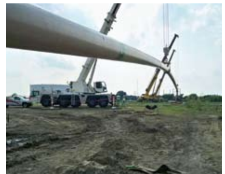
Figure No. 1 – Cranes support the product pipe as it transitions into the hole on the Elizabeth River HDD.
