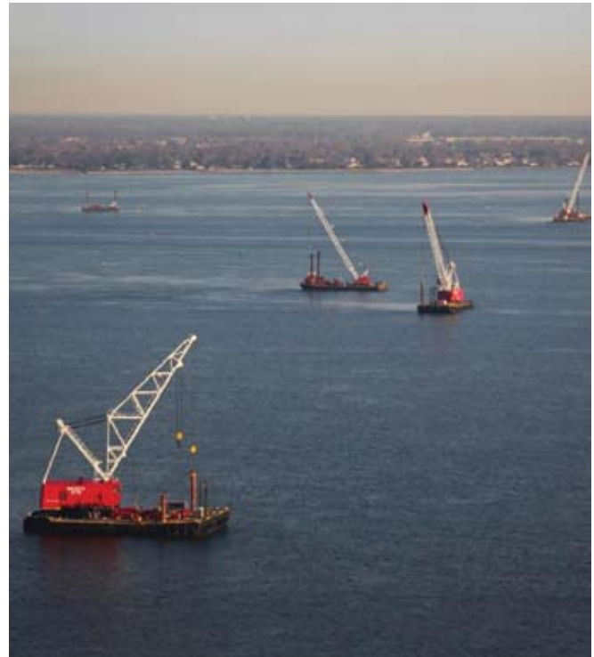
Figure No. 6 – An overview of the project depicting marine and HDD resources working at multiple tasks along the Hampton Roads installation route.
