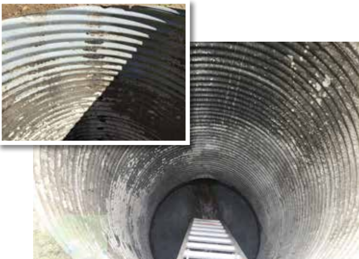
Figure 1. Existing bituminous coating deteriorating within riser structure
