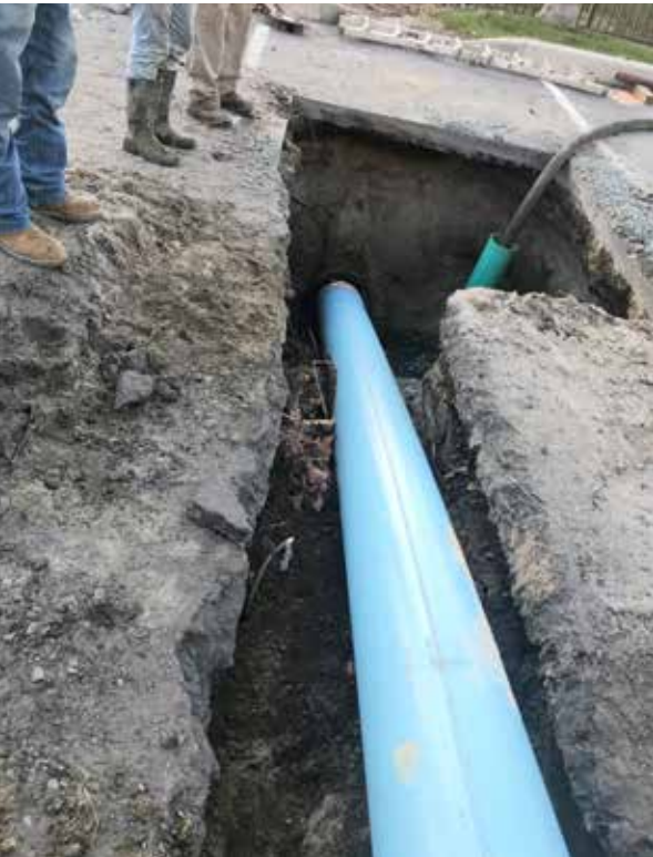
Figure 1. Pipe Burst in Process
