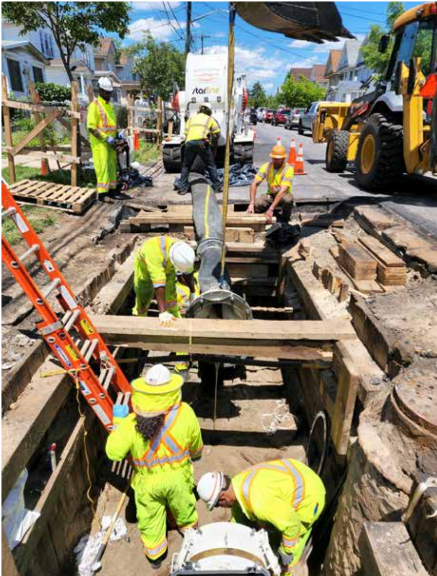
PPM crew prepare the transfer hose for lining the 24" cast iron natural gas pipeline
