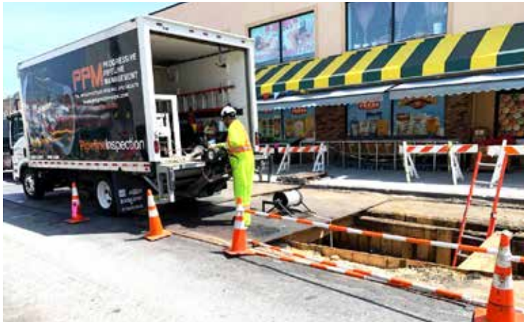
PPM crew with ARIES LETS CCTV camera used to inspect the pipeline prior to lining
