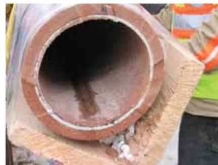
Figure 2. The invert of the CIP liner.
