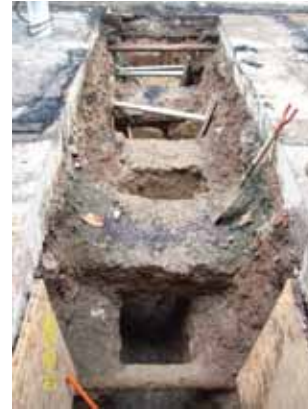
Figure 2. Numerous utilities were exposed to install just one sewer lateral.
