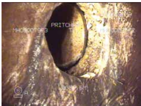
Figure 3 – Defective connection after 10 years of service with no CIPP degradation.
