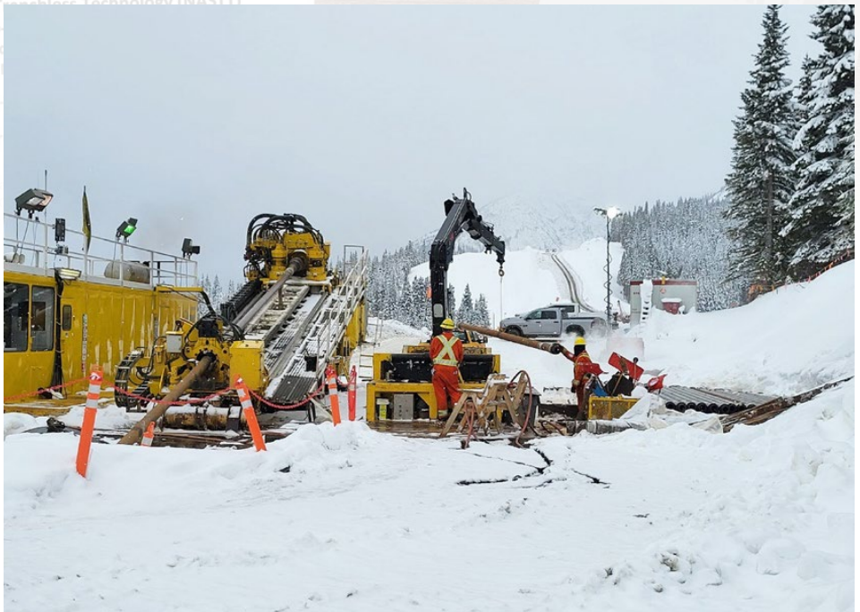
Figure 8. Geo-Pilot bore rig (during reaming) with pipe lay down area in the background
