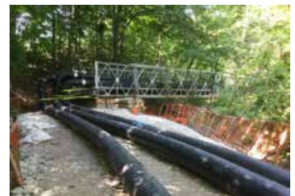
FIGURE 3: Bypass Piping and Creek Crossings.
