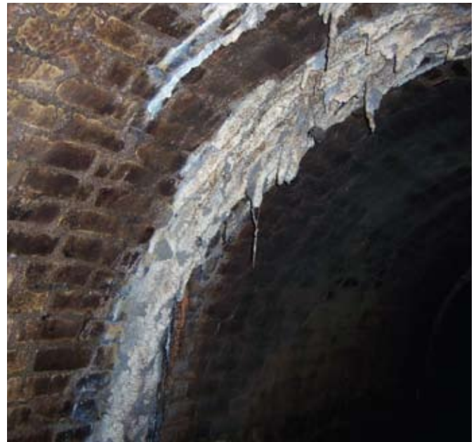
Figure 1: Mineral deposits reveal circumferential cracks in the brick arch.
