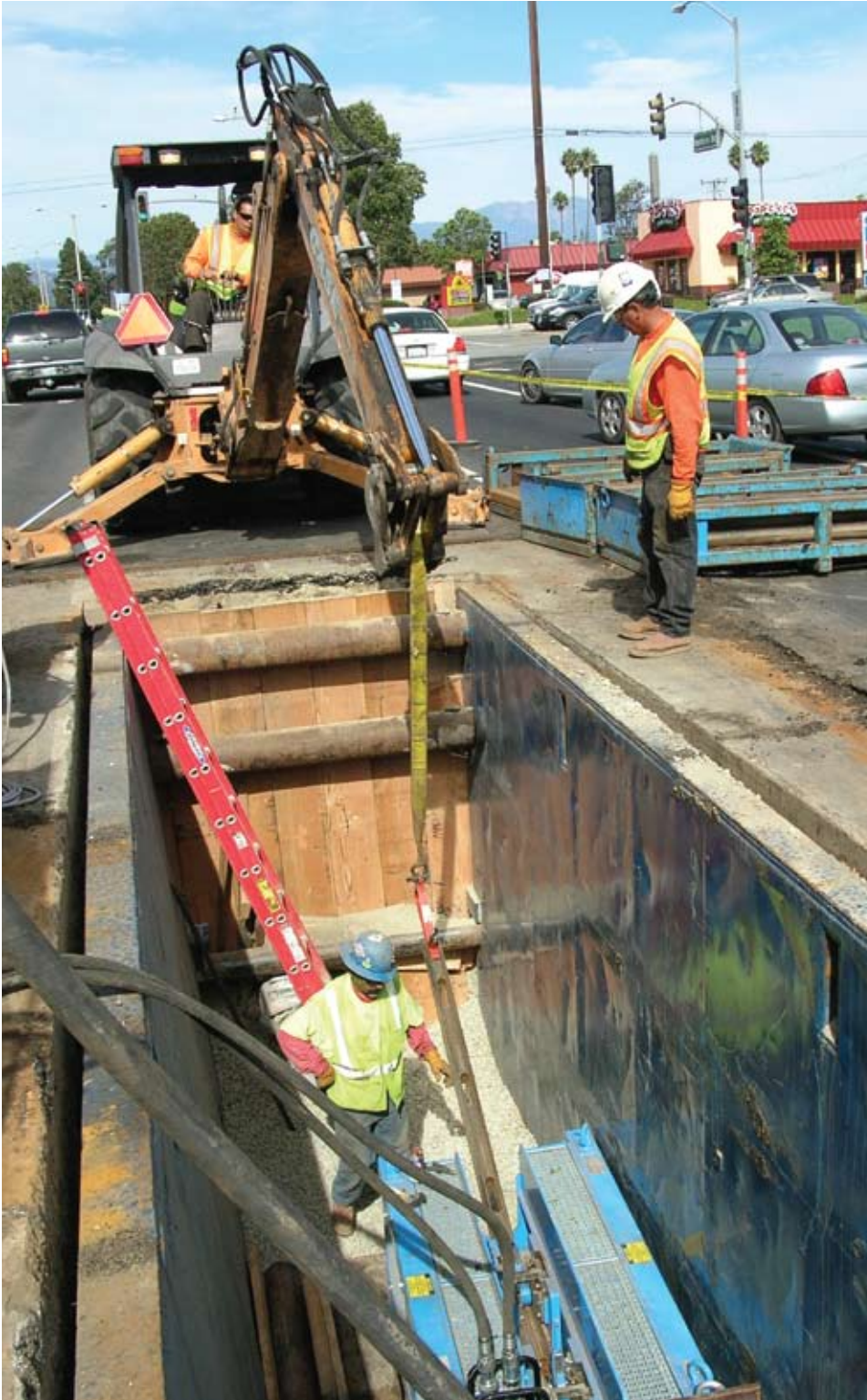
Crews utilized a Grundoburst static pipe bursting system with Quicklock rods, bursting 15-in. VCP and pulling in 18-in. HDPE.
