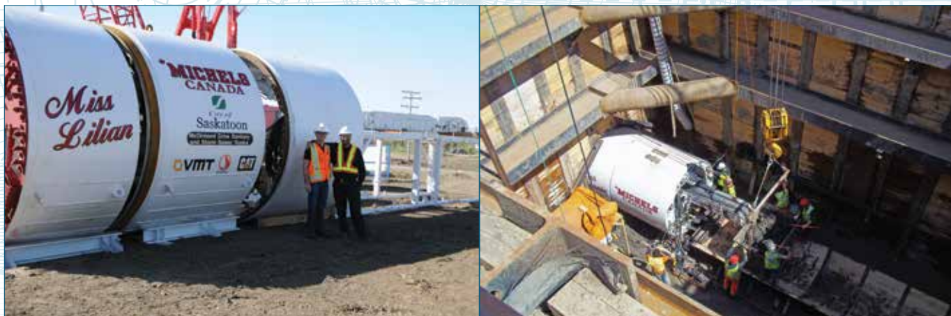
Figure 4 - Michels reviewed the two TBMs that were selected at the time of bid: a 2,280-millimeter (90-in.) Lovat EPBTBM for the sanitary sewer and a 3,275-millimeter (129-in.) Lovat EPBTBM for the storm sewer.
