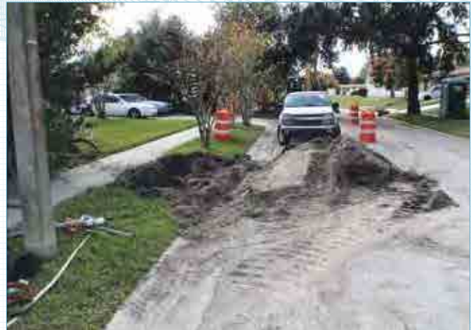
Bursting minimizes the amount of excavation on rehab projects versus traditional open cut methods. Impacts to developed neighborhoods and commercial areas with established landscaping are often minimized.
