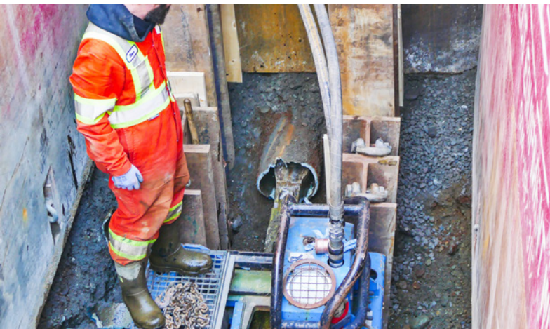
Removal of the large bursting head was complicated and required some extra excavation
