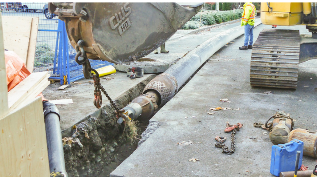
The large diameter HDPE pipe had to have a long sloped entrance ramp excavated to allow it to enter the host pipe
