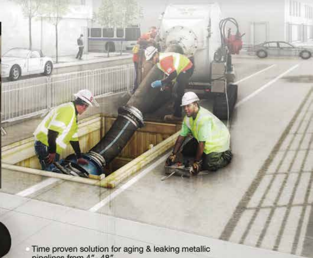
Largest gas main line in the world; 36" Cast Iron Pipe Renewal, Seton Hall, NJ, November 2017
